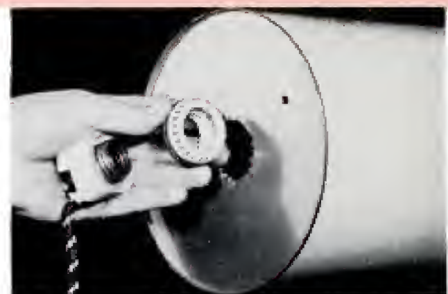
Above, two-piece porcelain socket of type used in signs is inserted in hole cut in bottom of can. Below, socket is protected by cover cut from small can. Metal tabs on can are drilled for metal screws
